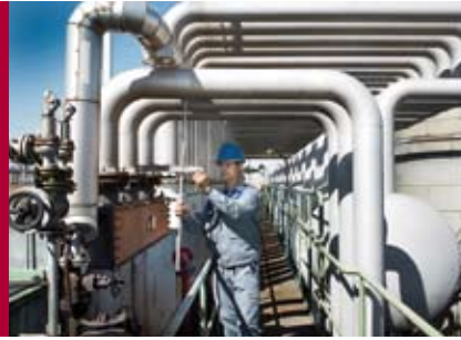
Planning, erection and conversion of piping systems – Voith Industrial Services can offer all the necessary services from a single source.
