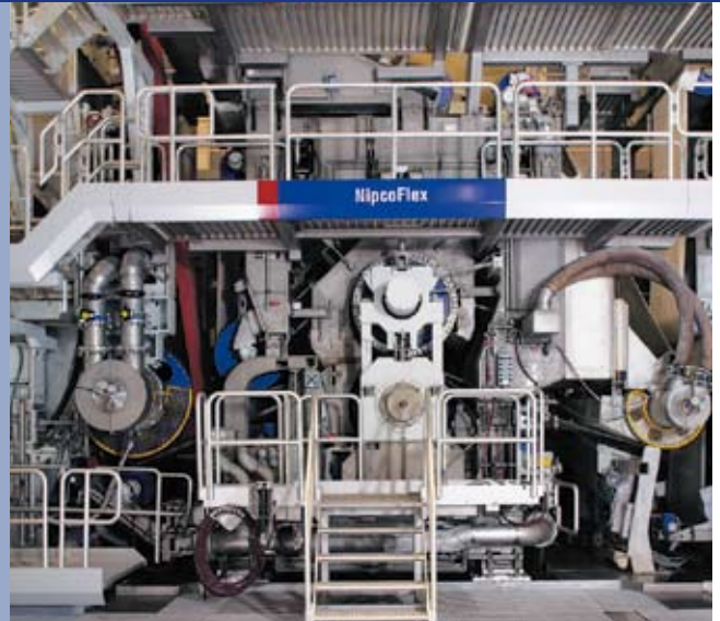
Press section of the Paper Technology Center in Heidenheim, Germany.
