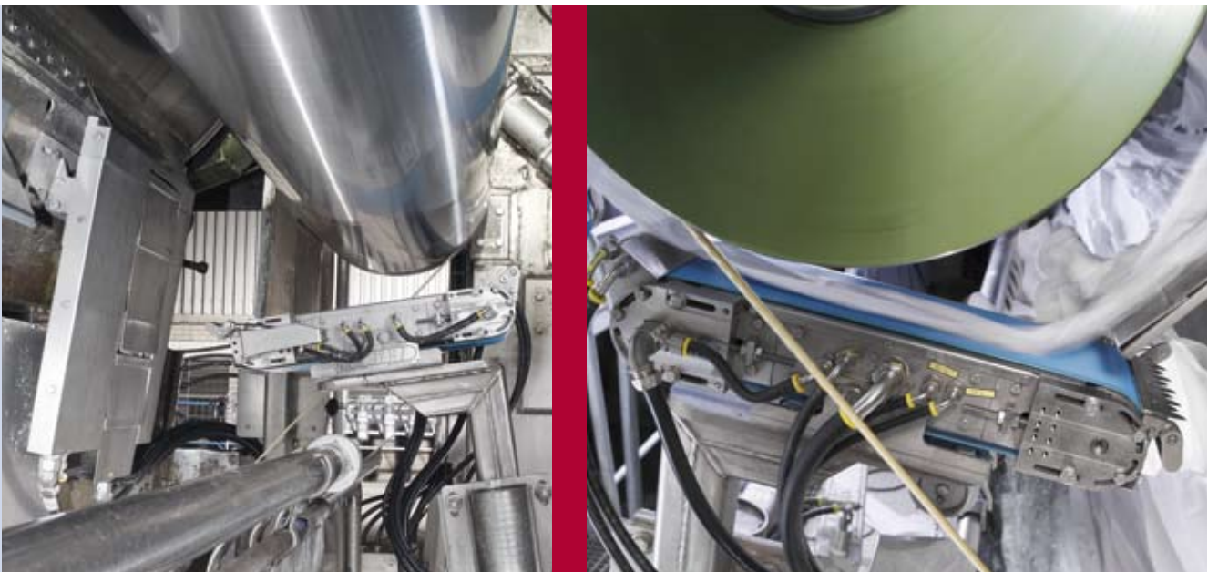
Fig. 4: Prevo threading solution on the PM in the SpeedSizer section (left: operating position; right: successful hit).
