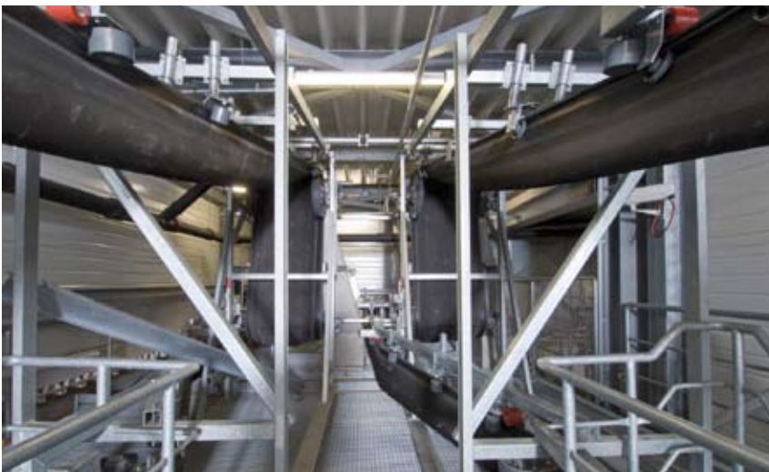
A closed pouch belt conveyor also allows fuel transport on complicated stretches.
