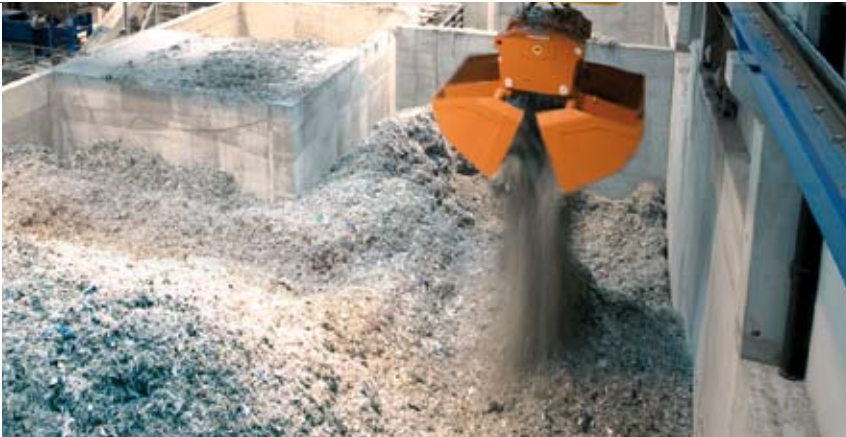
An intelligent self-propelled crane system takes fuel out of storage and feeds the secondary treatment stages, mixing and feeding systems.
